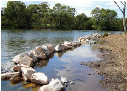
Rock fillets installed along the creek-bank to reduce erosion and promote mangrove establishment
